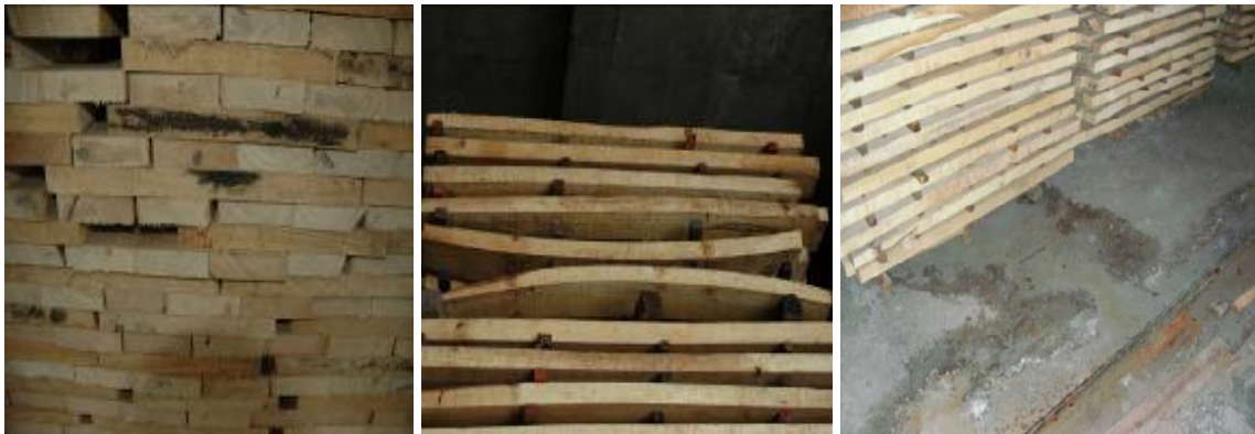
(21) (22) (23) Photos 21-23 (by Kim): improper stacking of timber inside the chambers
